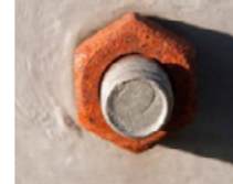
Example of Corrosion: Contact Between Dissimilar Metals
