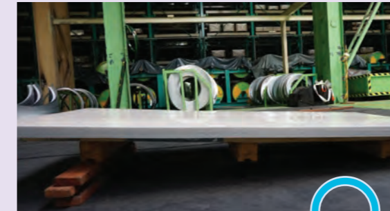
▲ Temporary measures when there is moisture inside the product
